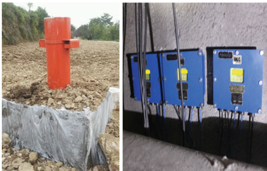
Fig. 5.13 Hydrological monitoring system (telemetry device and pipeline flow monitoring device)
