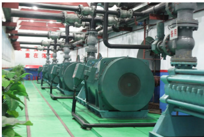
Fig. 5.10 Hujiache Mine central pump house
